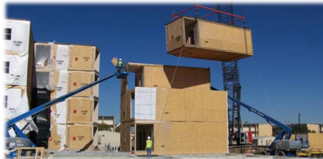
Figure 3 Modules lifted by crawler crane and stacked on top of each other
